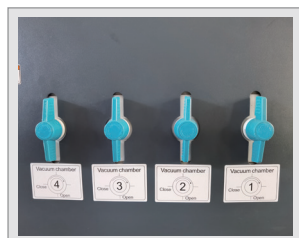
Vacuum Zone Control
